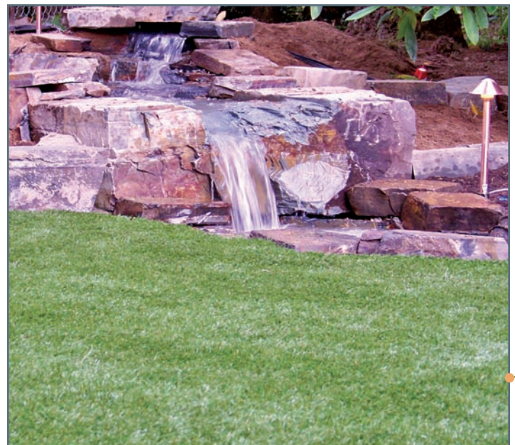
This recent installation featured a 25-year neglected yard rehabbed with water feature, terracing, new planting areas, lighting, and lawn.
